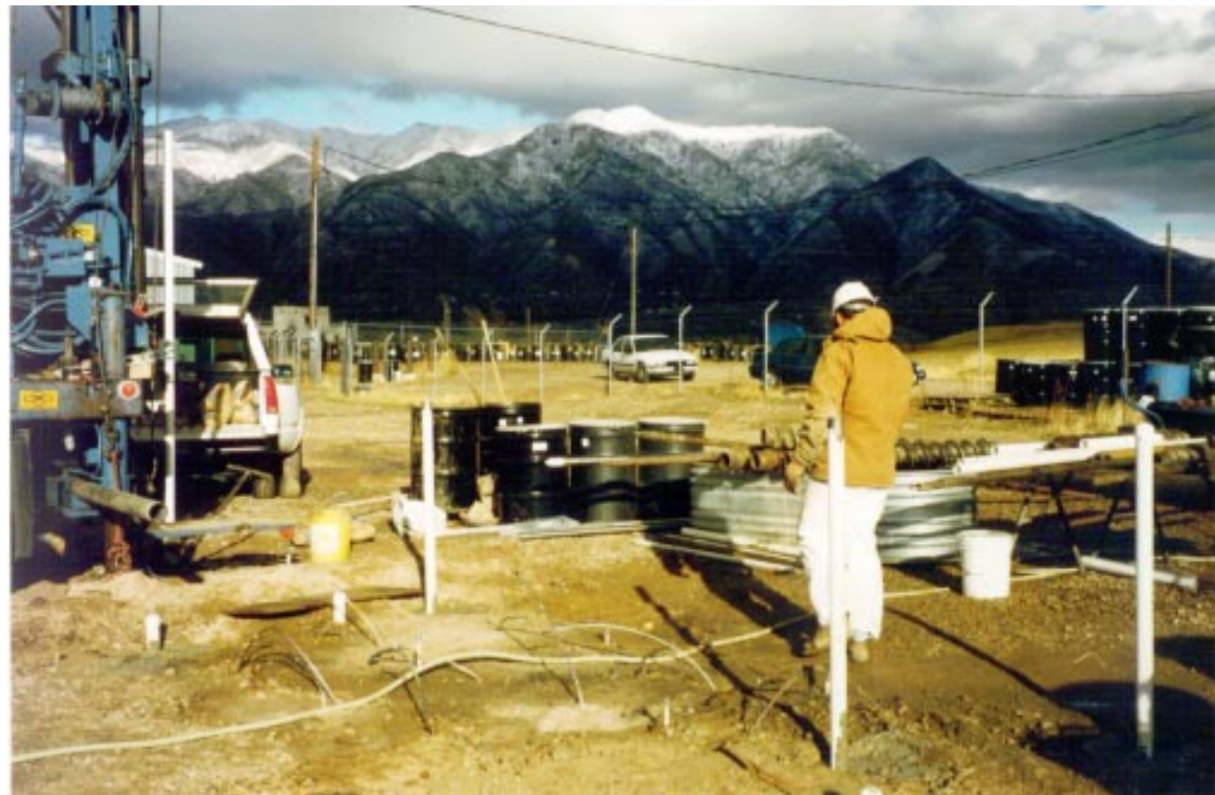
Installation of multi-level samplers and wells at the cosolvent injection site, Hill Air Force Base, Utah
